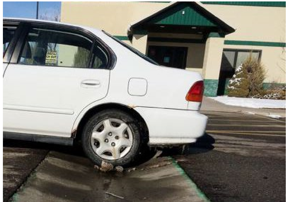
Road Surface Intact NOT Untreated Decay
