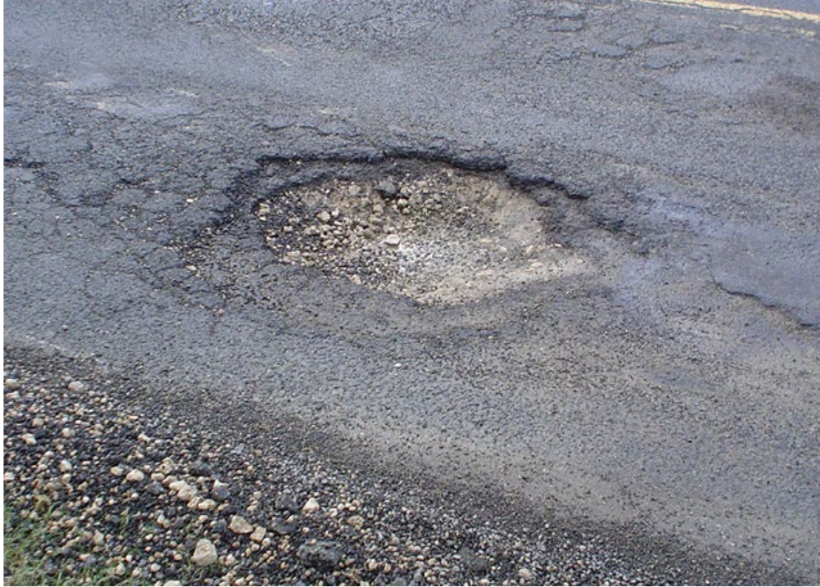
Definitive Hole in Road Surface Untreated Decay
